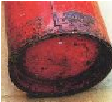
(層状はく離の腐食)
